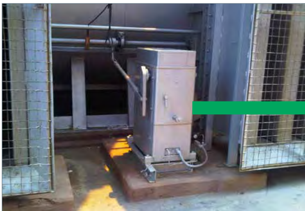
Before: Power station in Mexico where gas recirculation damper and FD inlet vane damper control systems are to be replaced.
