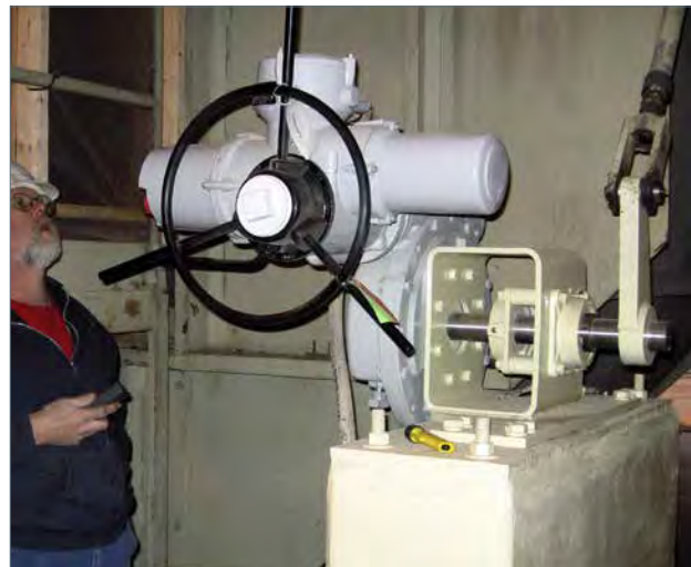
IQ Series on FD Fan Inlet Damper
