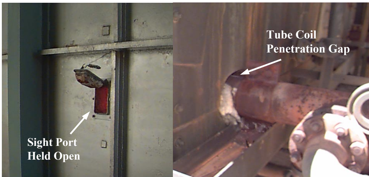
Figure 8 - Points of Furnace Air In-Leakage
