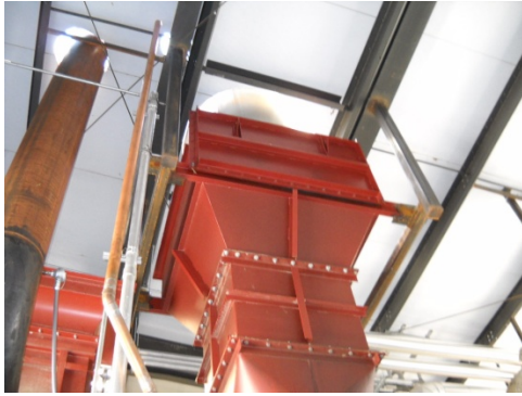
SCR on 50,000 PPH Firetube Boiler
