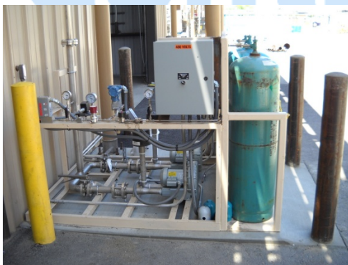
Ammonia Delivery Skid
