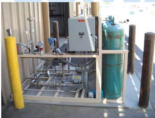
Ammonia Delivery Skid
