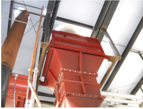
SCR on 50,000 PPH Firetube Boiler
